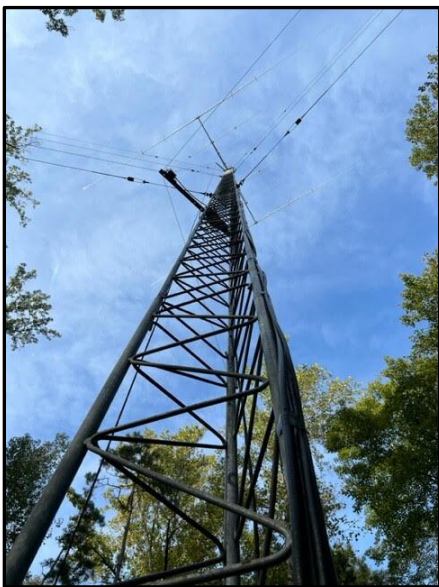
North Tower- C31, 2 ele 40, and elevated 80 ground plane
